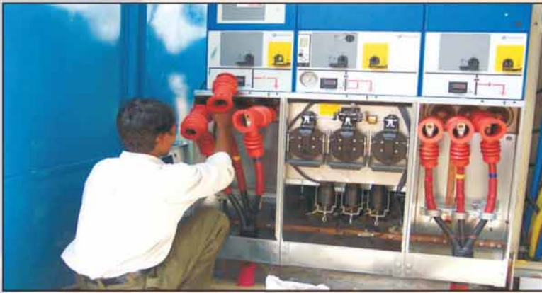
Installation of Silcab-T in ABB-Ring Main Unit
