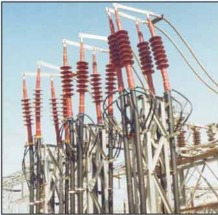
72kV Outdoor Termination installed in West Bengal Development Corporation Ltd., Bakreshwar
