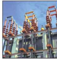
Raychem Heat Shrinkable Termination installed in Switchyard
