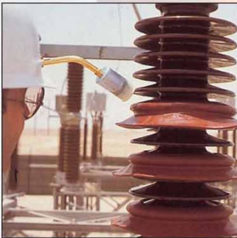
Raychem's Creepage extender installed on a insulator
