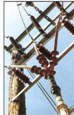
Raychem 33kV termination installed on Surge Arrester which also functions as a support insulator
