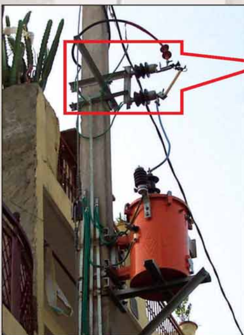
D.O fuse before insulation
